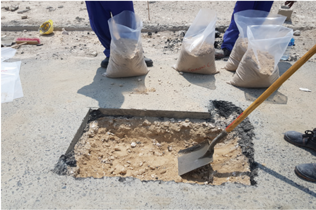
Figure 6-2 Exposed subbase after 4 years in service – EW material
