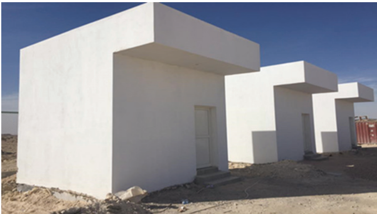
Figure 5-10 Trial buildings, 6 months after construction: control (100%) gabbro on left; 50% Wadi gravel in centre; 100% Wadi gravel on right.
