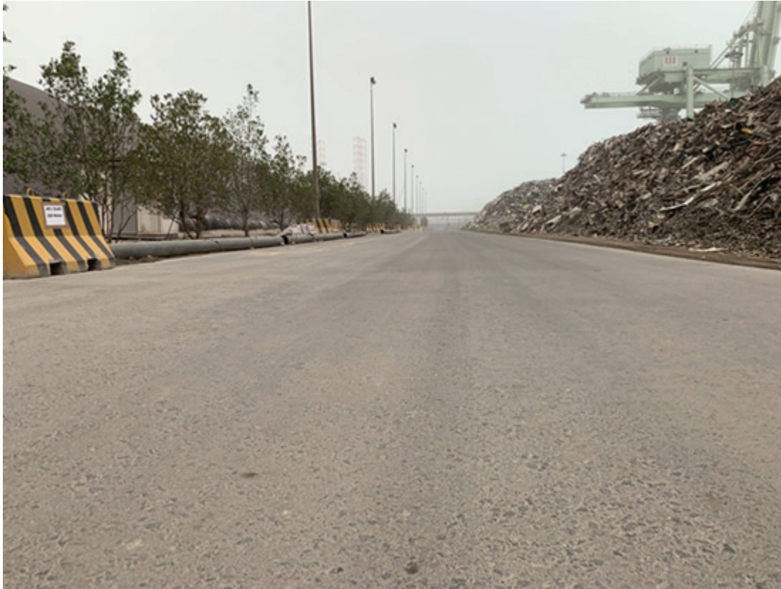
Figure 4-9 Visual condition of the pavement trials after 3 years in service
