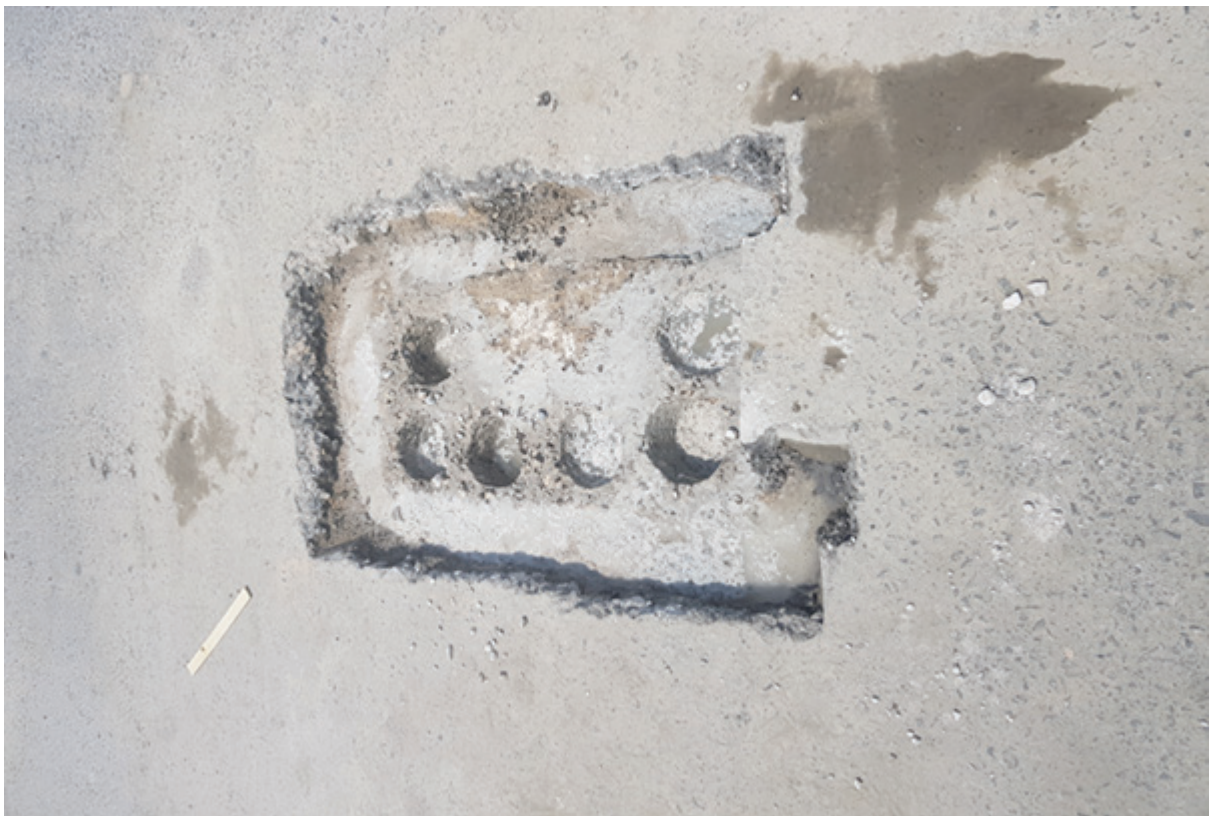
Figure 6-3 Exposed subbase after 4 years in service – RCA material
