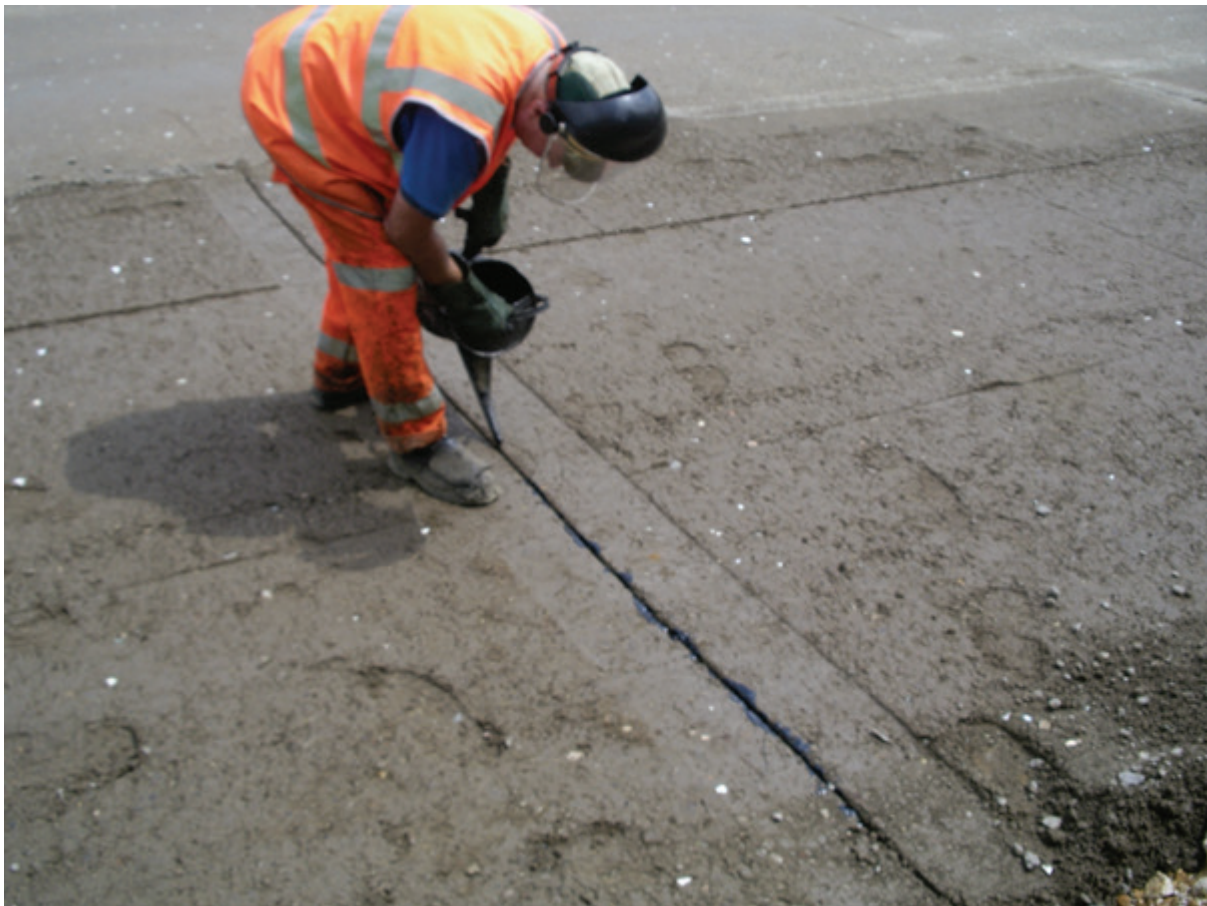
Figure 6-13 Induced CBM cracks and filling the grooves
