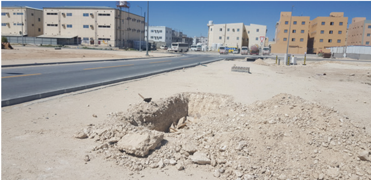
Figure 7-8 Exposure of granular materials under footway, adjacent to a carriageway
